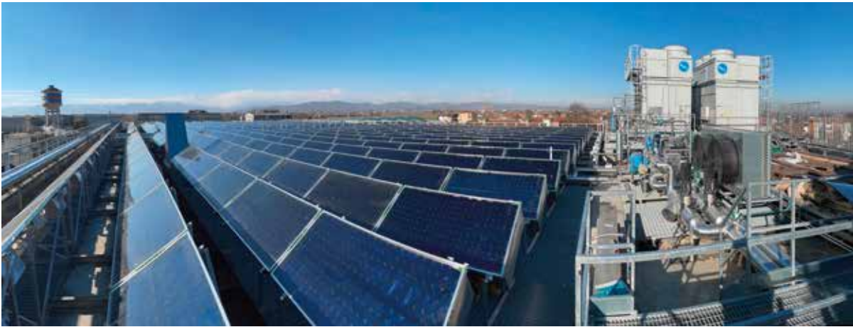
Solar process heat system for Martini & Rossi with a capacity of 0.42 MW th and equipped with high-vacuum flat plate collectors in Turin, Italy Photo: TVP Solar, Switzerland
