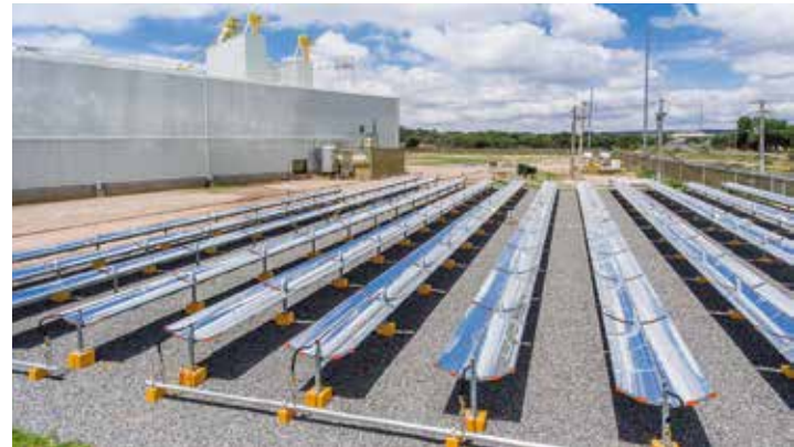
Parabolic trough collectors installed at Comercial Forrajera de Lagos (COMFOSA) in Mexico
