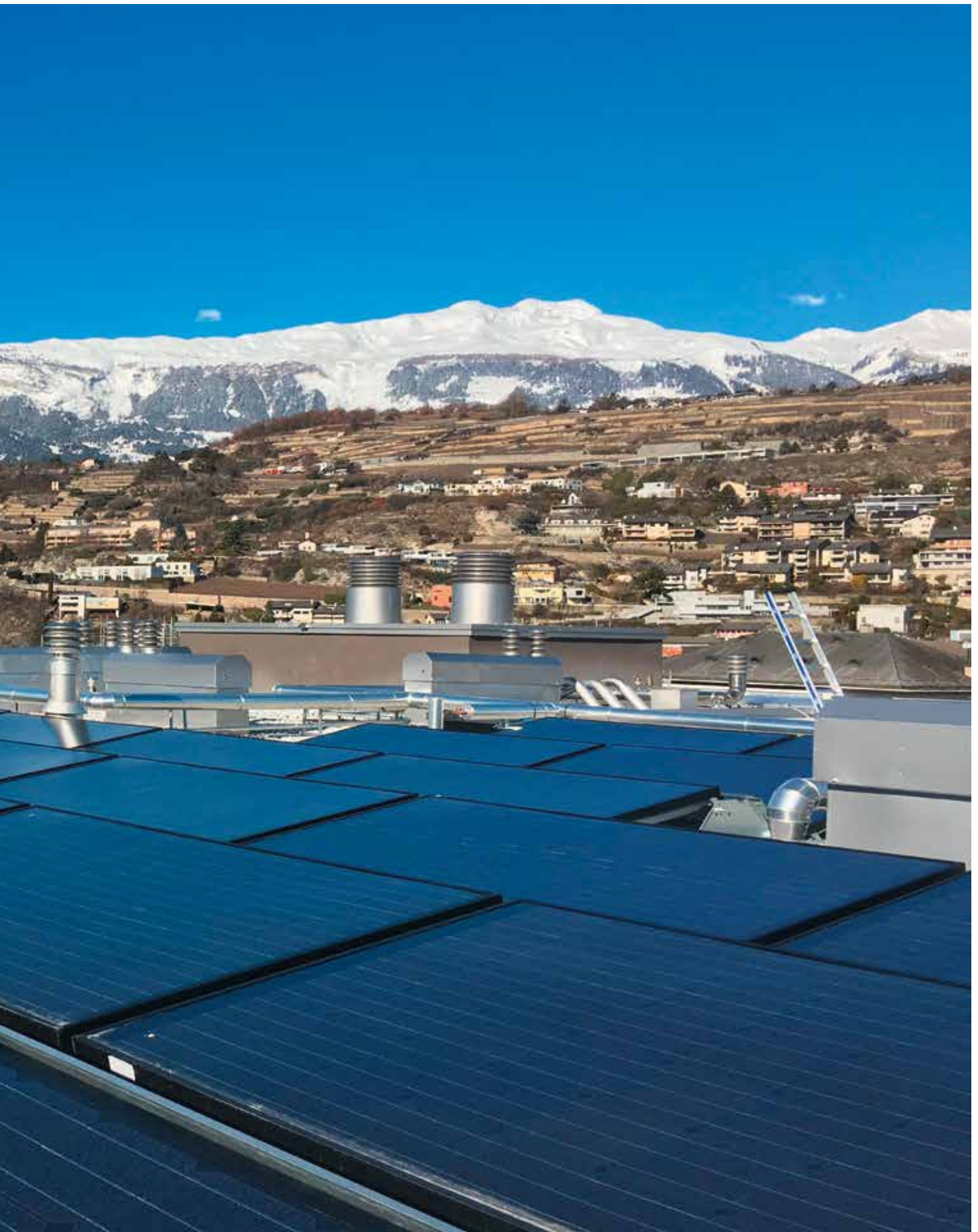
Sion, Switzerland. 41 PVT collectors on a building in the city center (sustainable building with Minergie label) Photo: DualSun, Switzerland
