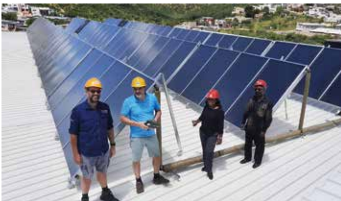
Partial view of the solar installation on Lady Pohamba Hospital in Windhoek, Namibia Photo: AEE INTEC
