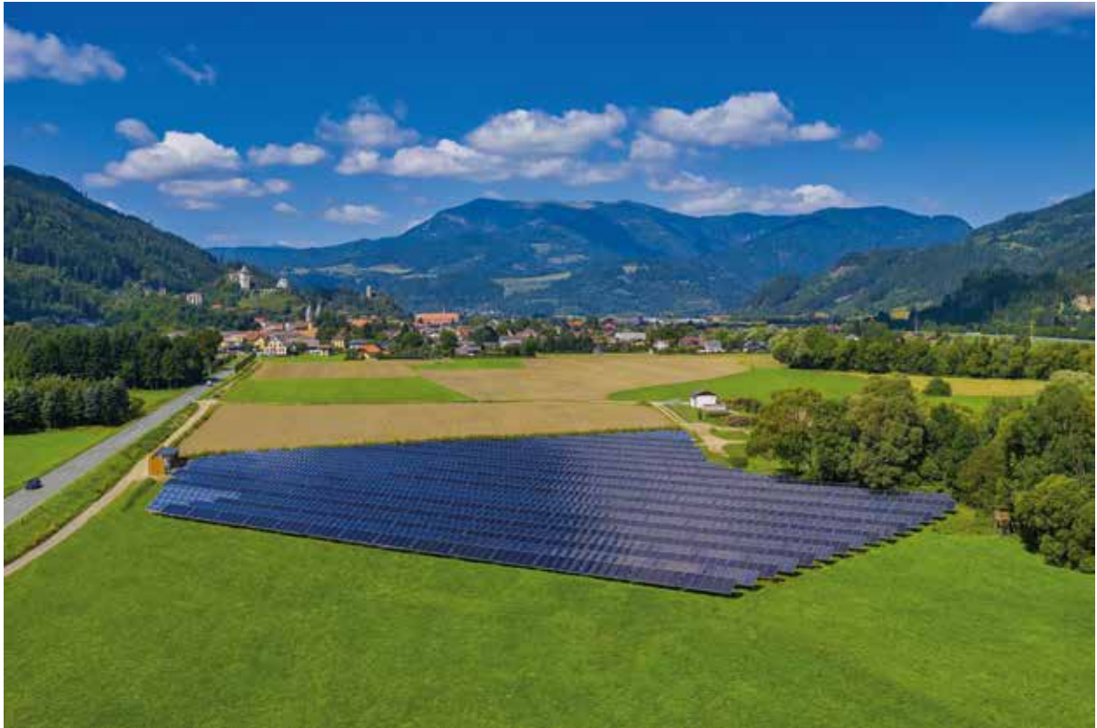
The Austrian solar district heating system in Friesach, with a capacity of 4.1 \text{ MW}_{\text{th}} , corresponding to 5,950 \text{ m}^2 flat plate collectors, was installed in 2021 Photo: Greenonetec Solar Industry GmbH, Austria
