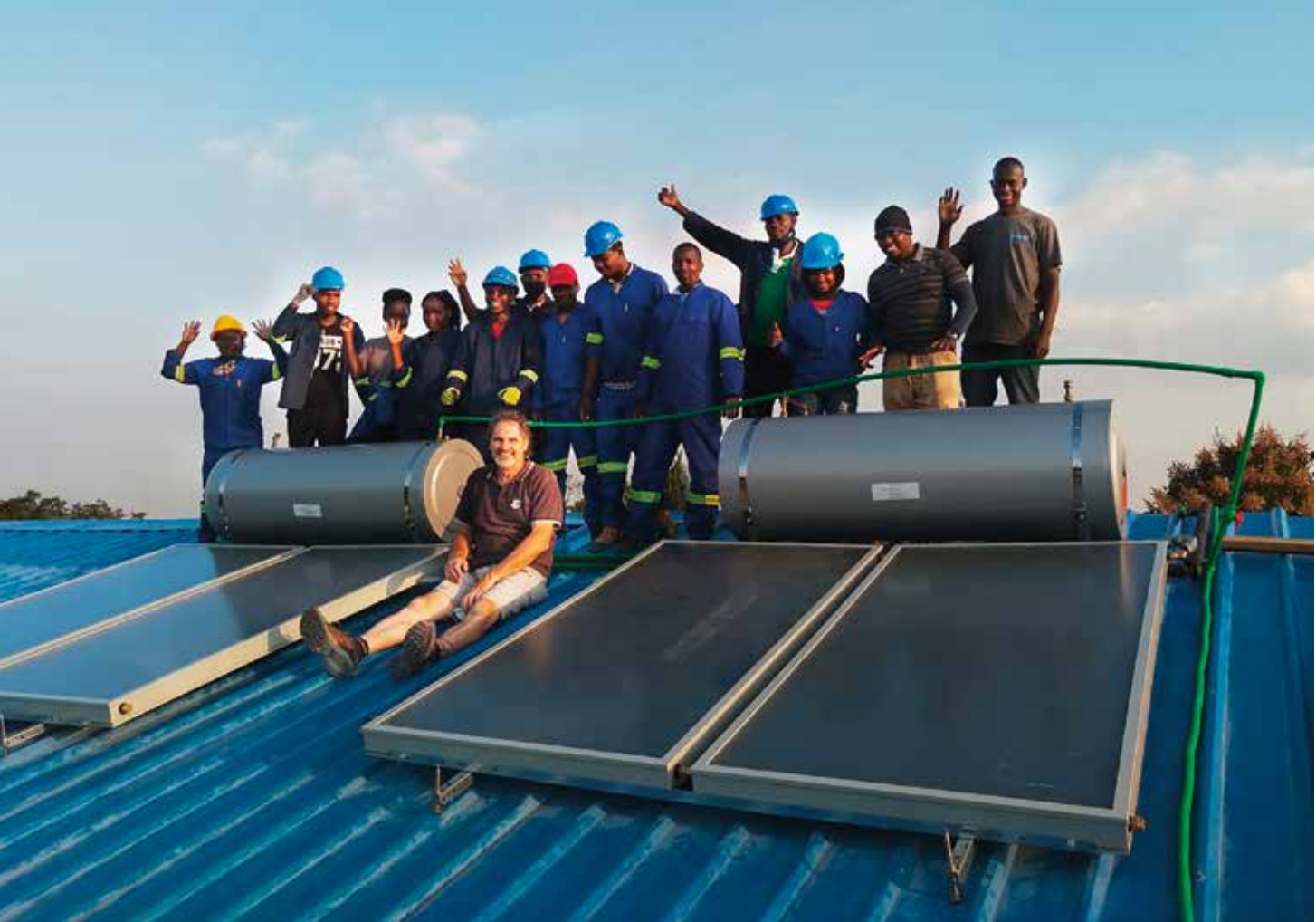
Thermosiphon systems in Mozambique
