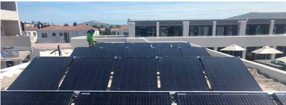
High-temperature PVT system at Windtown Hotel in Langebaan, South Africa. 27.5 kW thermal and 7.6 kW electrical combined with a 19 kW heat pump
