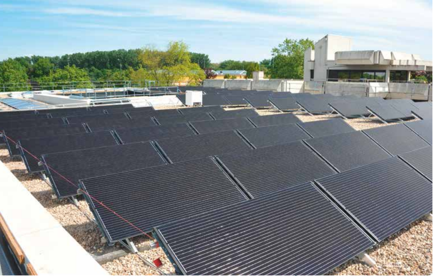
200 m 2 PVT-collector field for a new office/council building in Offenbach an der Quaich, Germany Photo: Consolar, Germany
