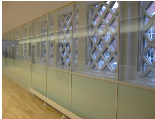
The old façade was preserved by adding floor-to-ceiling glazing on the inside.
