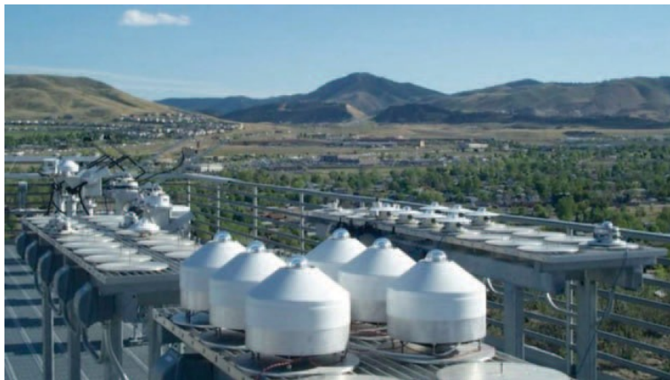
Figure 3-10. Kipp & Zonen model CM22 pyranometers installed in CV2 ventilators. Photo from NREL
