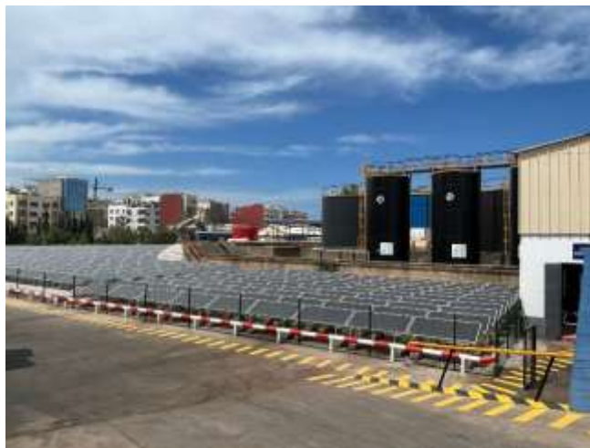
Figure 5 1,750 m 2 high-vacuum flat plate solar field: Photo Credit: TVP Solar
