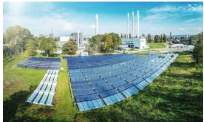
Figure 4 Fernheizwerk Graz, collector test field with 3 different solar thermal technologies from 7 different manufacturers: Photo Credit: SOLID Energy Systems GmbH
